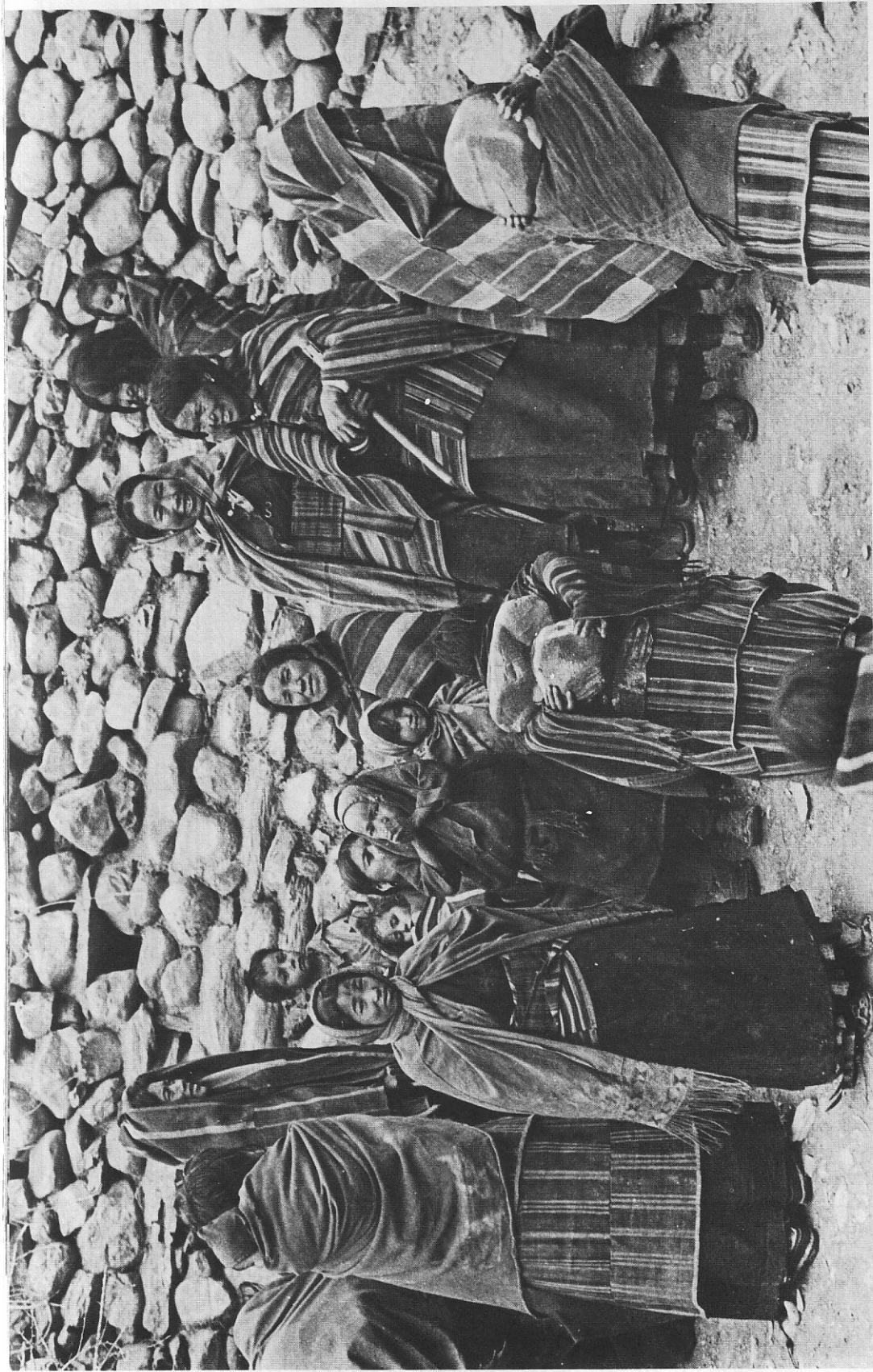
A group of women repairing the retaining wall of a communal water canal. Men and women normally work together on collective projects, but in late autumn, after the India-bound migrants have left the villages, most of the work is done by women.
