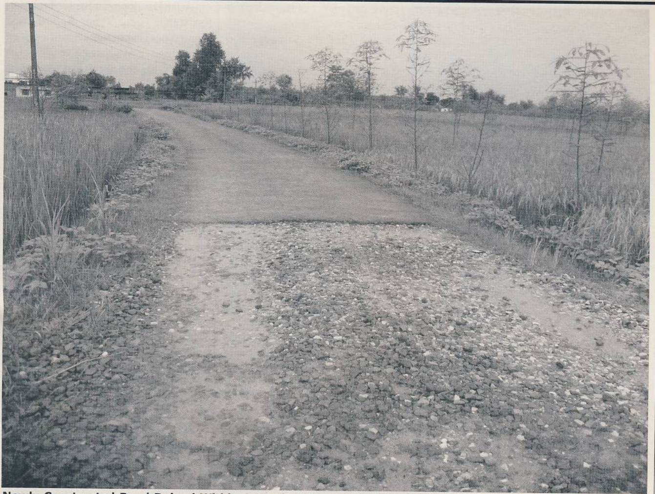
Newly Constructed Road Ruined Within A Week : Misuse of resources
