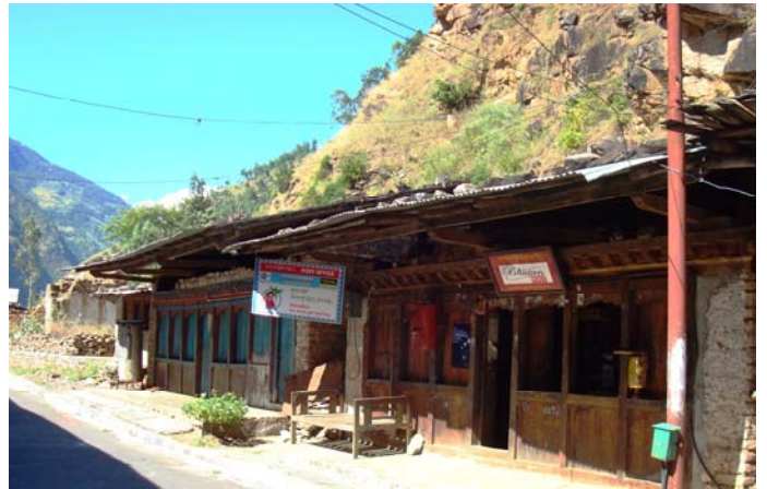
The neighboring houses of the PO have been ruined by the rock fall
