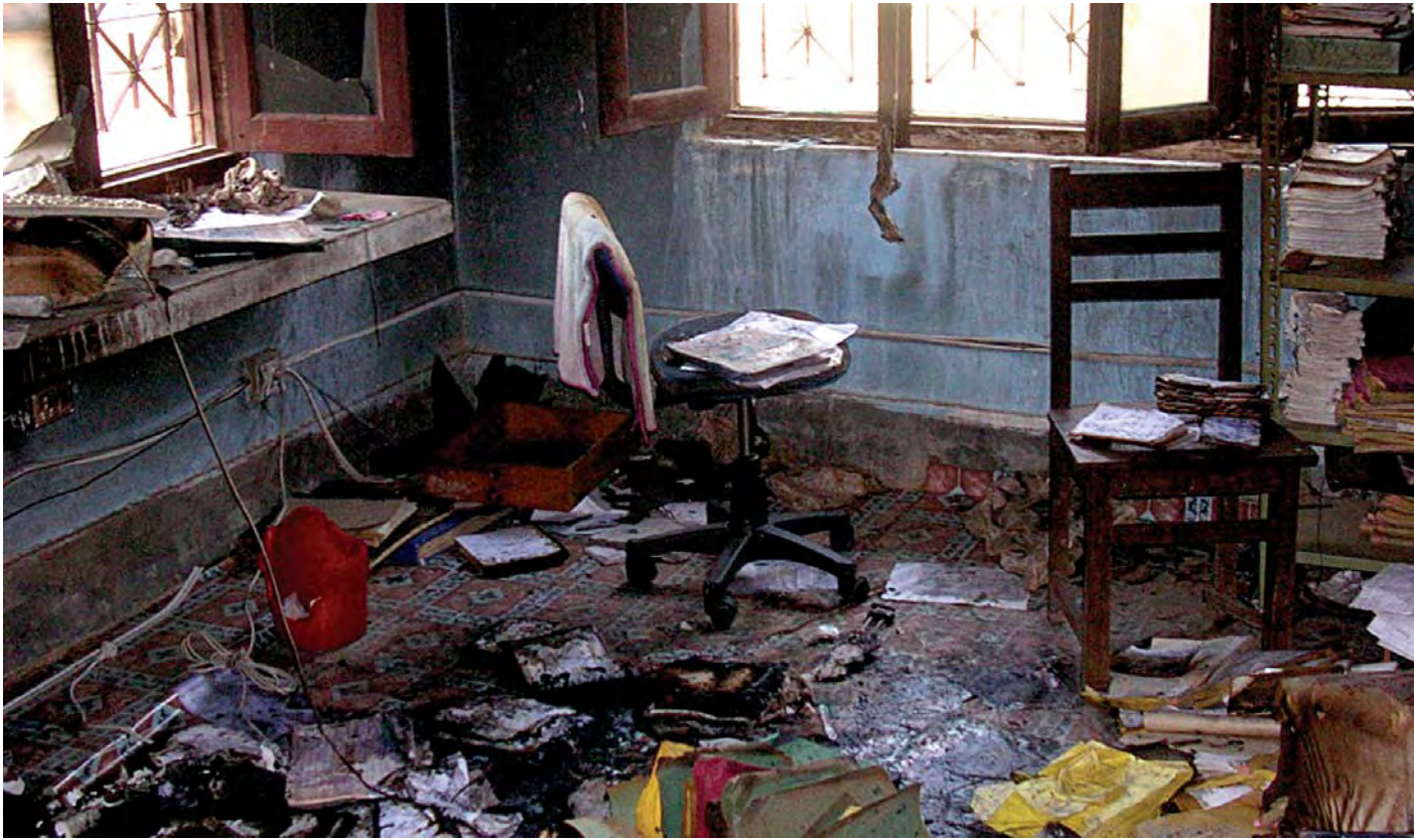
YCL set fire engulfs Land Revenue Office in Berdia
