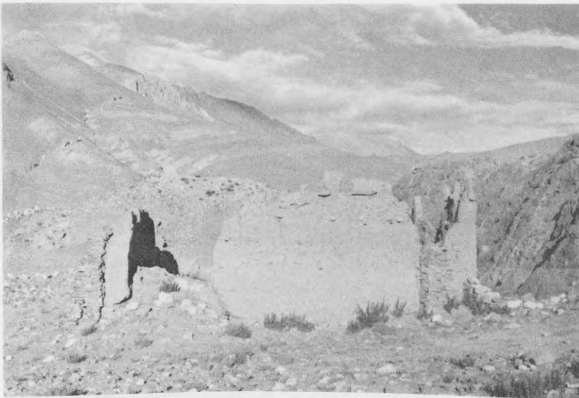
P-10 Phyug-'tsho Grog-po rDzong. Note the walls of adobe and stone sandwiched together.
