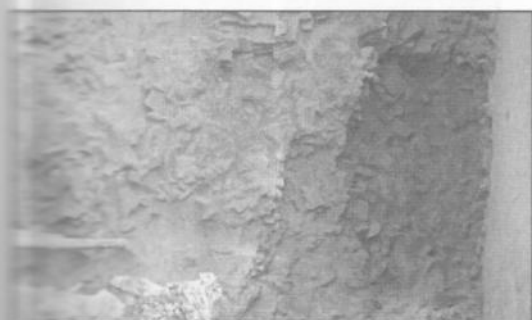
P.No.71 Fallen debris of bricks at G5(IV)
