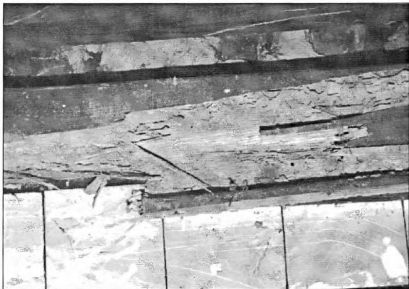
Wooden Portion attacked by Termite
