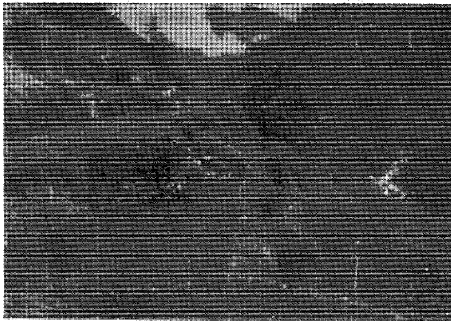
Plate No. 1 - Bank collapse
