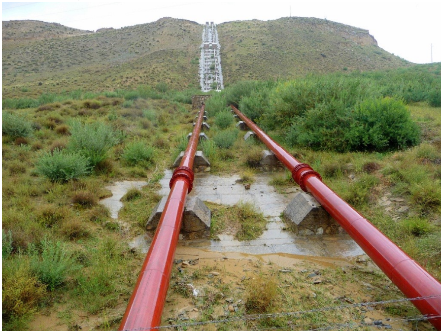
Photo 99. Pipes from a reservoir move water to a cistern.
