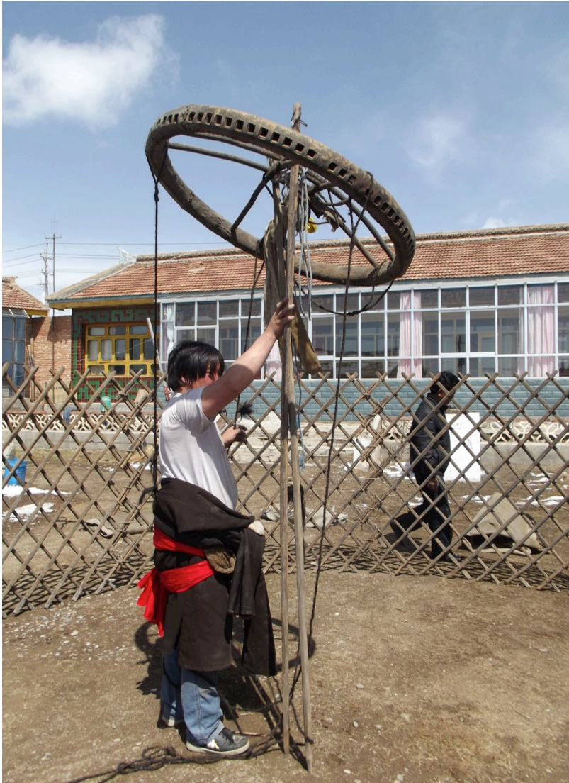
Figure 19. Preparing to raise the skylight in the center of the yurt frame.
