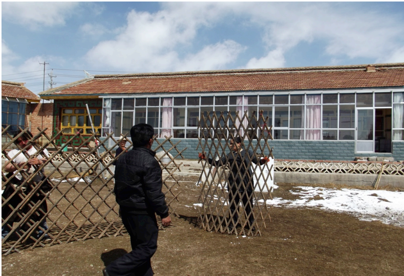
Figure 17. Setting up the lattice panels. The man (left) ties two panels, and the woman (right) will join the panels.
